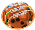
Wiring conductors in a flush-mounted junction box.
